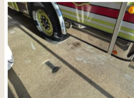
Insufficiently sized floor drain in apparatus bay.
